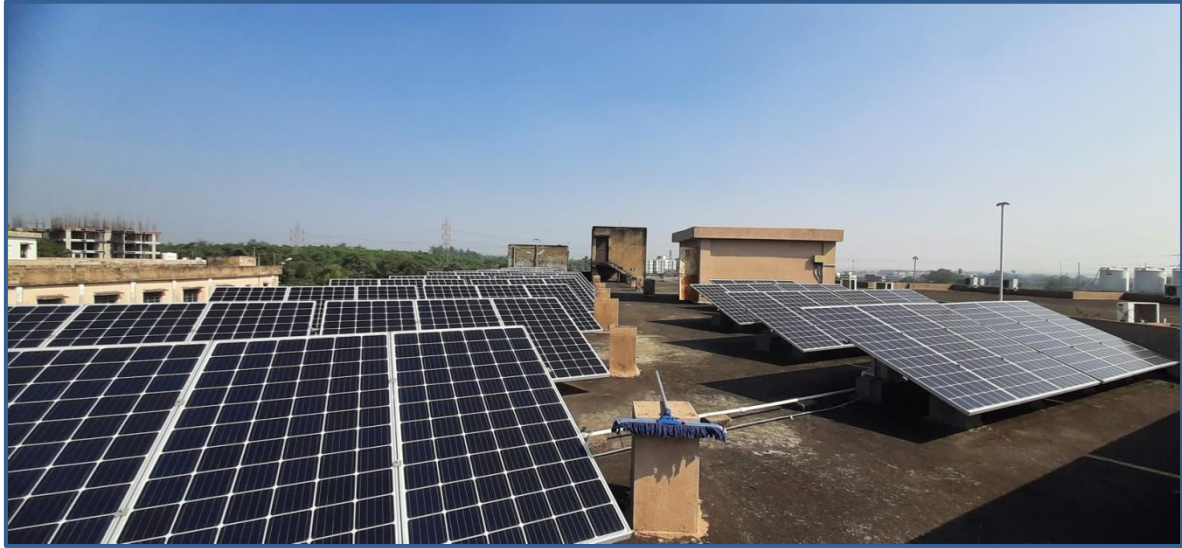
30kW On-Grid Rooftop Solar Panel
