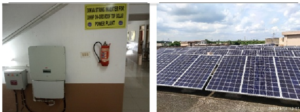
Fig. 9.11a: 30 KW solar power system
