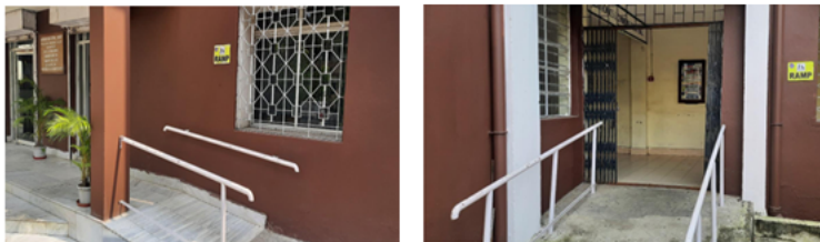
Fig. 9.12d: Disabled-friendly ramps at campus
