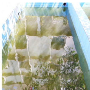
Fig. 9.11d: Rainwater storage tanks.
